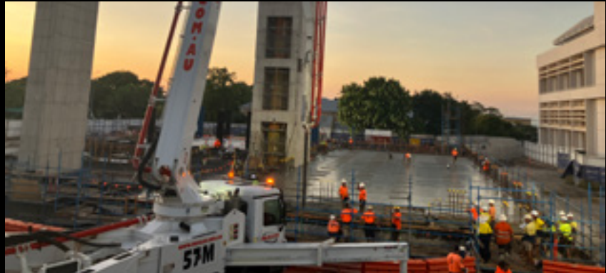
The construction team completes the concrete pour for the suspended concrete floor slab of Gallery 1. Image: by Josh Griffin, Projects and Precinct Site Manager, Department of Logistics and Infrastructure, 6 June 2024
